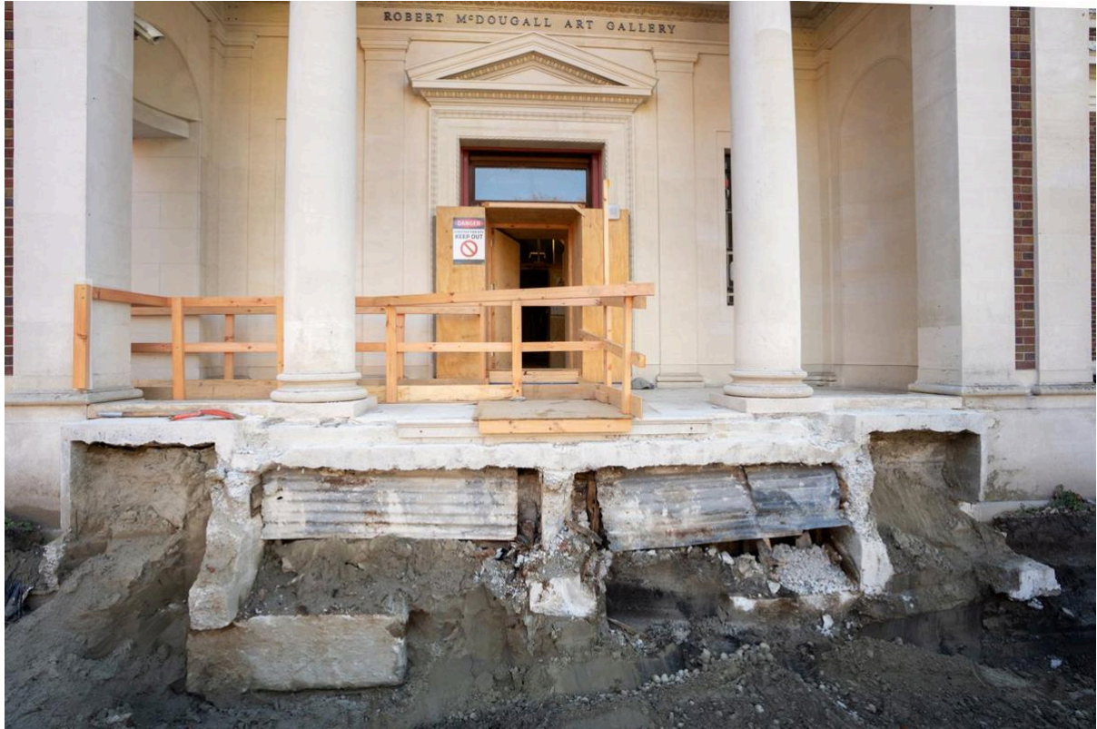
Contractors are preparing to demolish and excavate out the old Robert McDougall Gallery basement.
