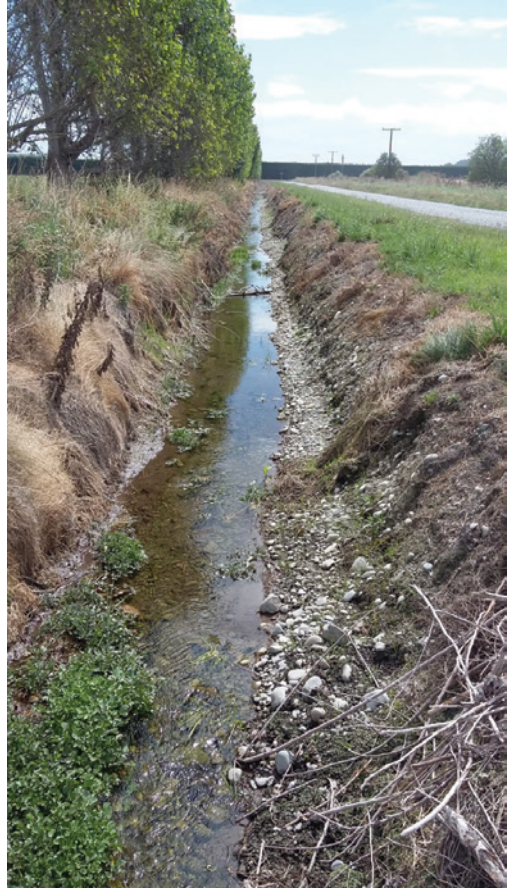
Figure 2. Boyd Road drain. March 2019. McEvedy collection
