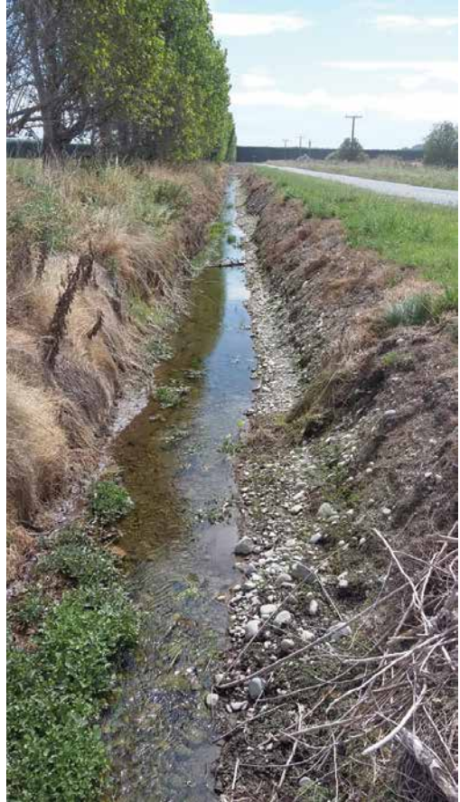
Figure 2. Boyd Road drain. March 2019. McEvedy collection
