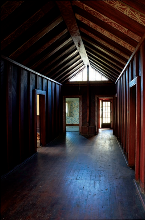
Figure 6. Rehutai Hallway showing the key elements in Māori architecture: central ridge pole painted with kōwhaiwhai (curvilinear) designs, heke (exposed rafters) also with kōwhaiwhai paintings, which lead down to pilasters performing the role of poupou (vertical rafter supports). Photograph: D Smith, 2012
