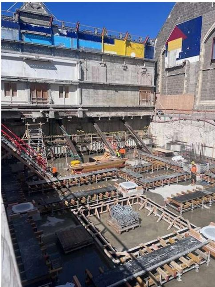
Zone 1 Base Isolators and Grillage
